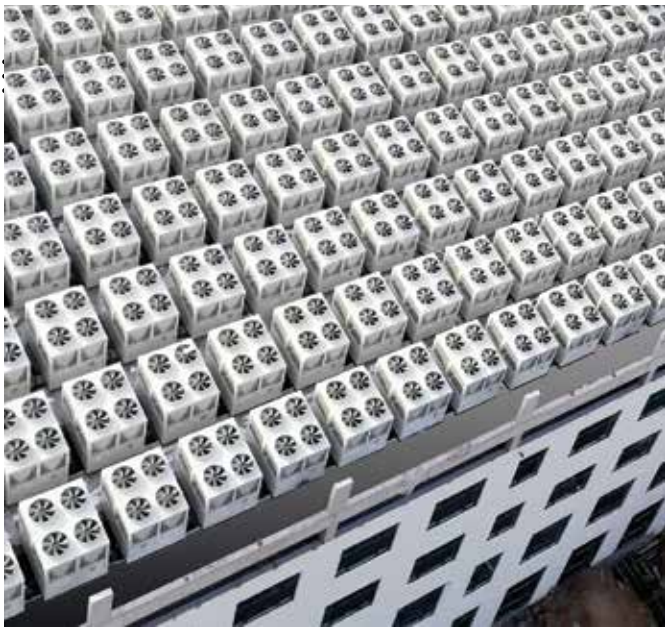
Figure 3: More than 1200 units of ASHPs were deployed as heating sources for approximately four million square meters of living spaces in large residential buildings. The challenge was how to best distribute these units and move the heat from the ASHPs to the living spaces.
