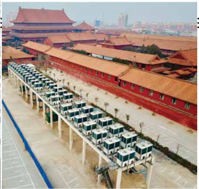
Figure 4: The “cold island” effect occurs if the air circulation around the ASHP units is not optimized. In this case, all the stations were designed as frame structures at least eight meters above the ground.
